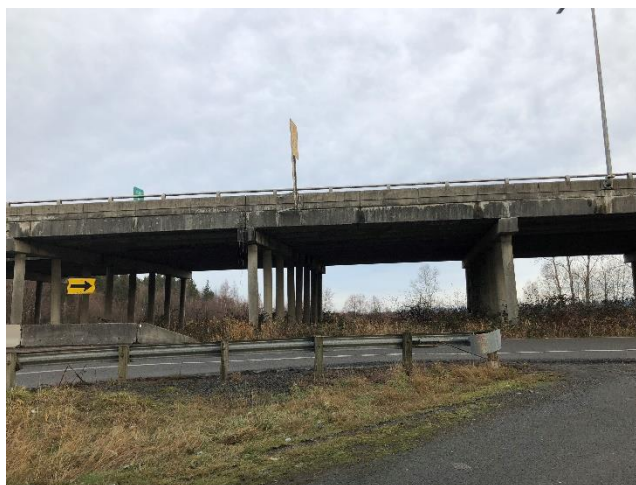
Picture of the underside of the US-2 westbound Trestle, showing the bend in the pillars
